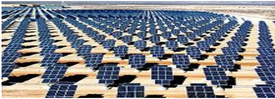
Fig-3 A 14 MW Power Plant in Nevada, USA Installed in 2007
